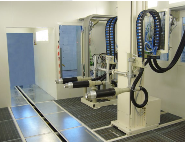
Example of installation (INSA plastics laboratory – France)
